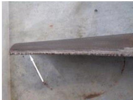
Figure 1: Leading edges of steam turbine blades where damage due to drop impingement erosion is most significant
